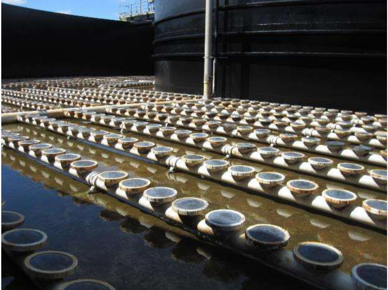
Figure 15. Diffusers for air in the activated sludge basin
