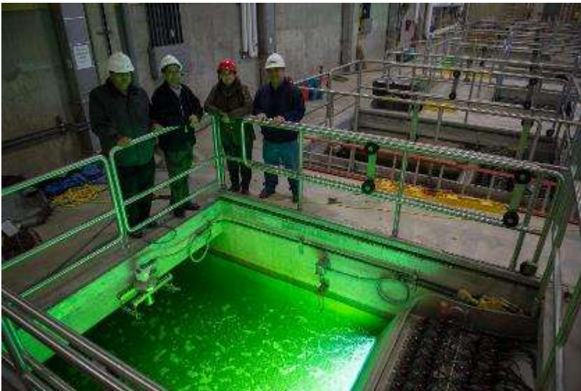
Figure 39. O'Brien wastewater treatment plant UV disinfection units. (MWRD 5/11/2018 presentation at Fermilab)
