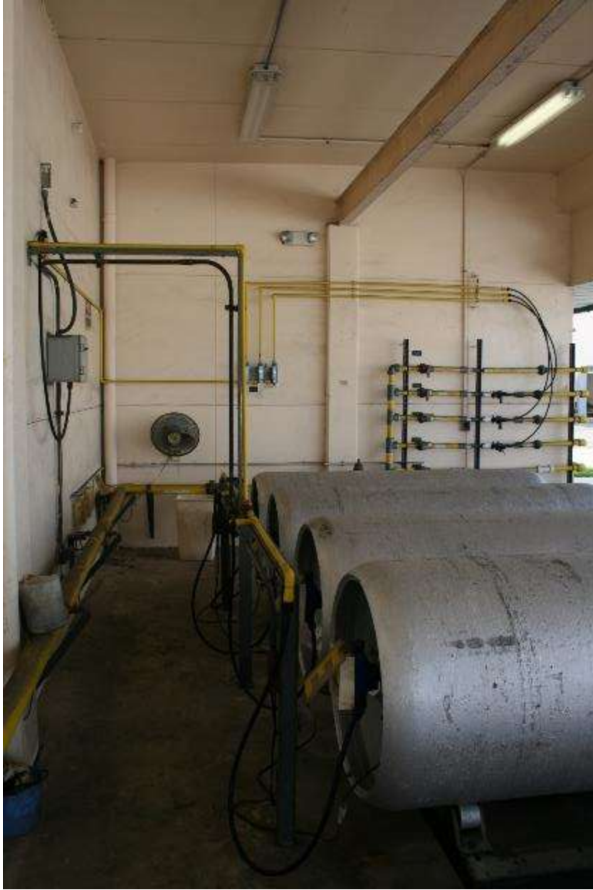
Figure 20. Chlorine cylinders (gas)
