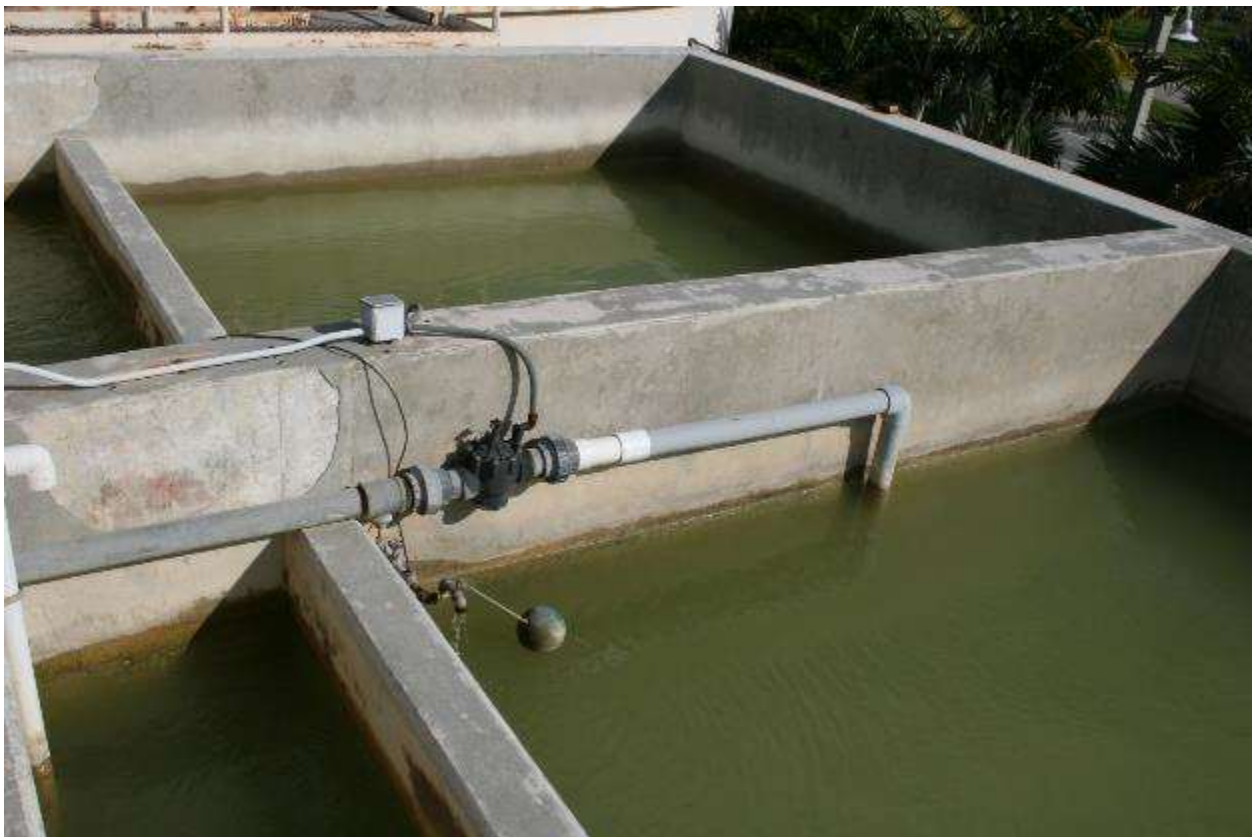
Figure 22. Typical gravity sand filter
