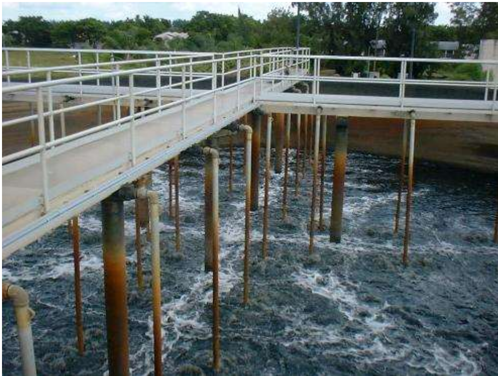
Figure 13. Aerated, primary clarifier, also used for flow equalization
