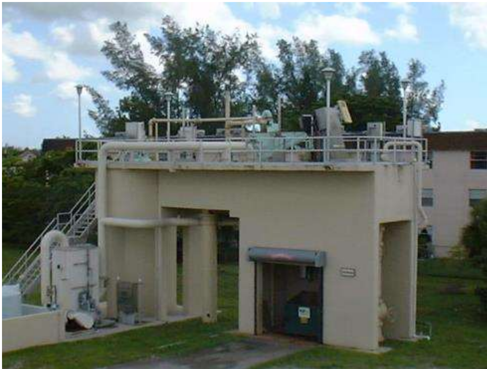
Figure 12. Bar screen and grit chamber at the headworks of a WWTP
