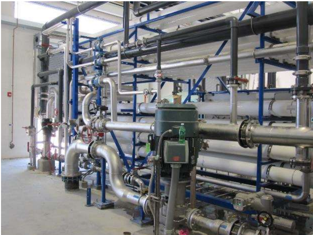
Figure 27. Installed reverse osmosis system
