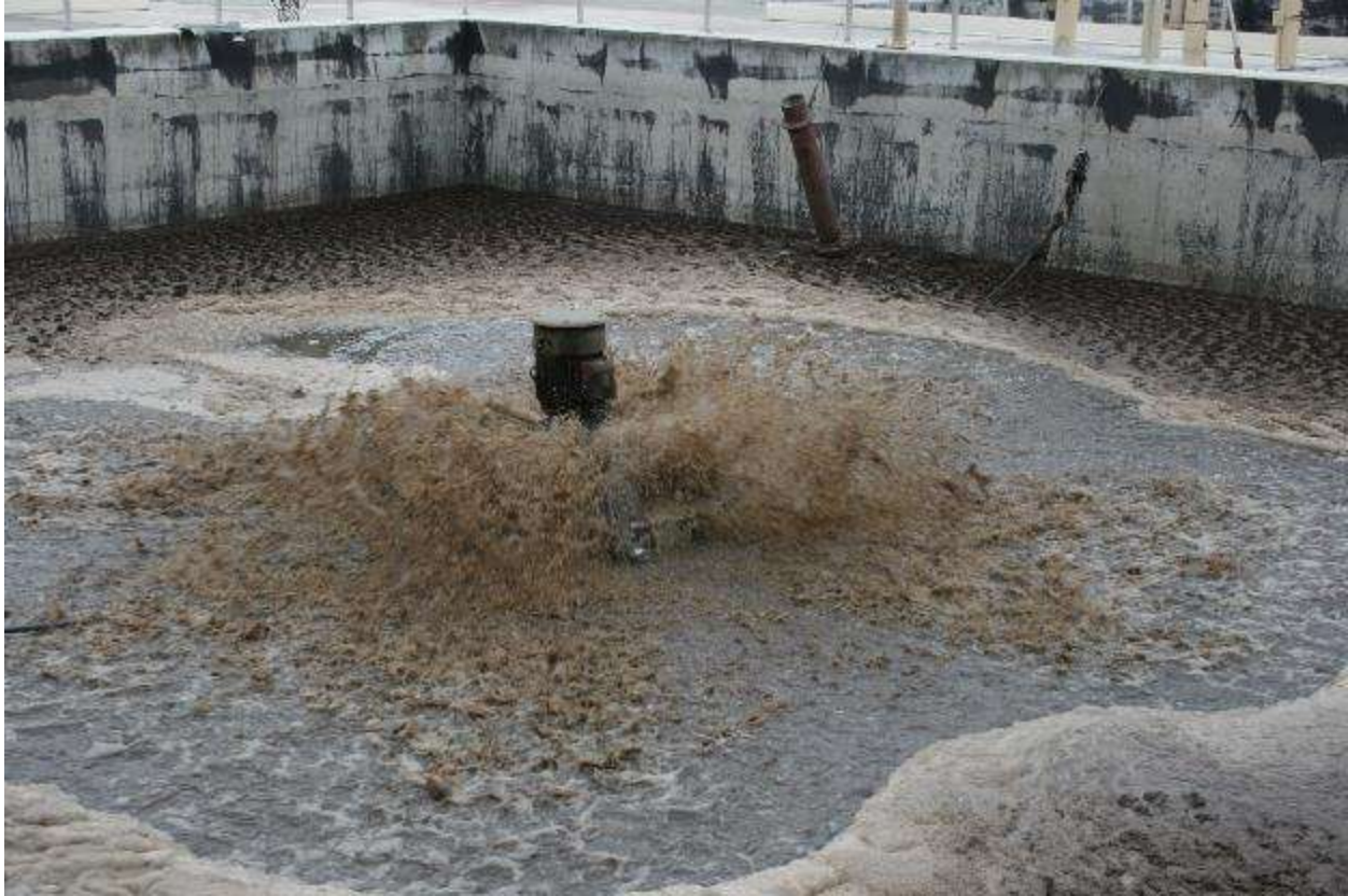
Figure 16. A mechanical mixer or sparger for adding air to the WWTP
