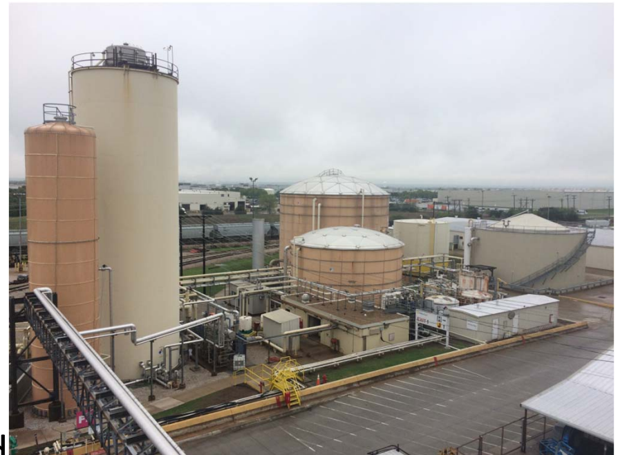
Fort Worth wastewater treatment
