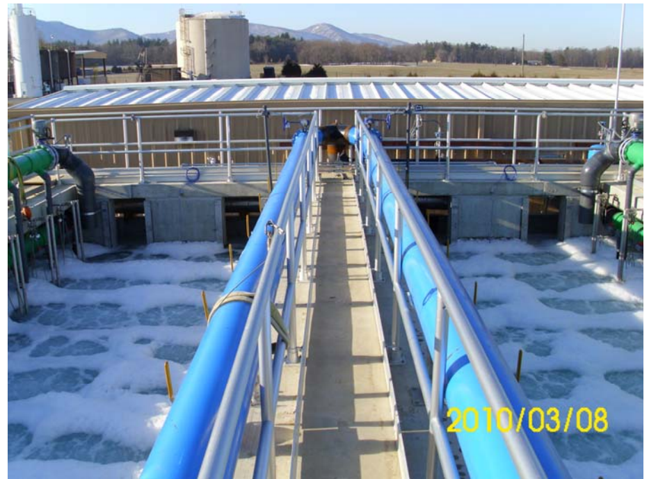
Shenandoah wastewater treatment
