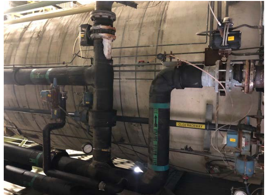
Fort Worth Water treatment
